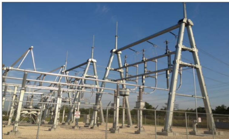
Figure 6-3. A Station Training Yard with a Control House and Equipment
