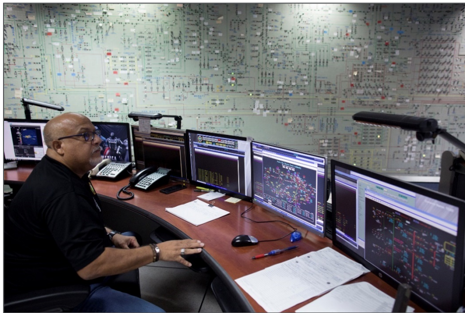
Figure 2-2. Monacillo Control Center
