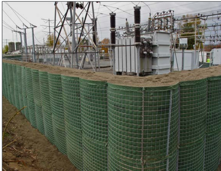
Figure 4-6. Substation Flood Barrier
