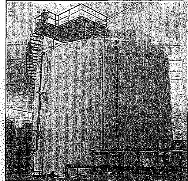
PREPA Effluents Tank
