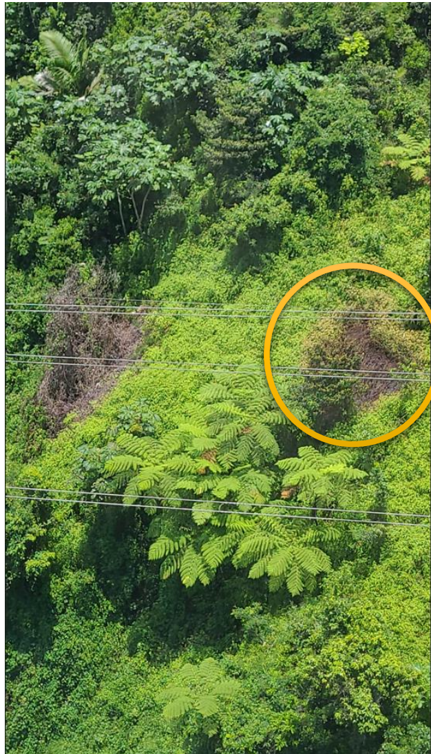
Figure 3-2 Burned Vegetation at the point of the fault in Line 50700 from Yabucoa to AES
