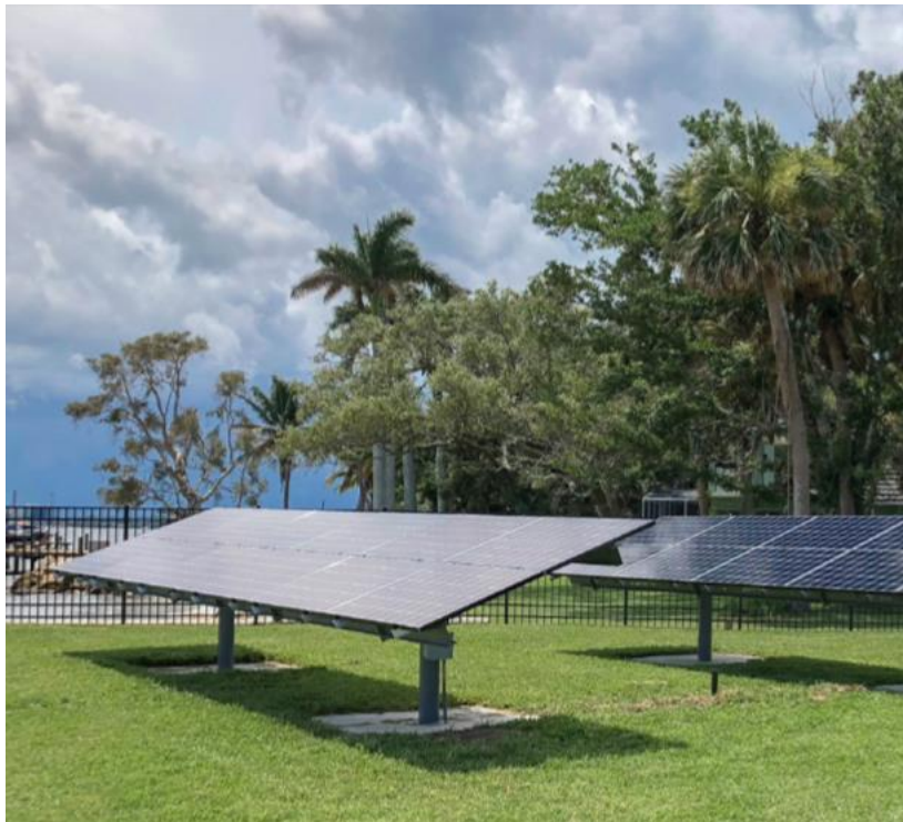
Figure 11: Prefabricated Solar mounting of PV
