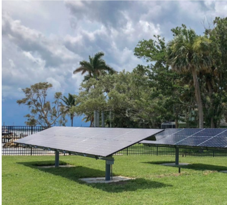
Figure 7: Typical ground-mounted canopy style PV system in open fields.
